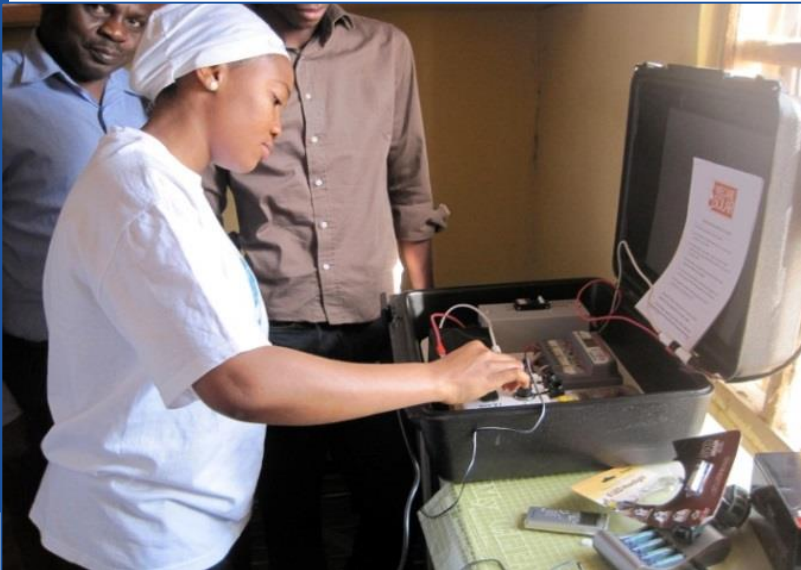
Solar suitcase powering a health care facility in Nigeria.
