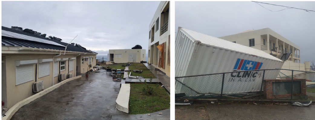
Celina Clouden Smart Hospital, west side view (l) and home for doctors and nurses (r). Photo credit: Ton Vlugman PAHO WASH Consultant
