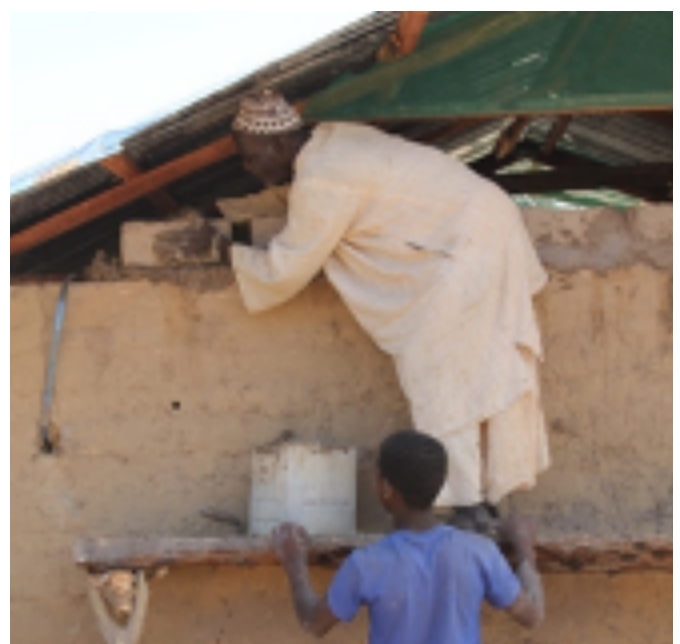
Closing Eave Gaps in the Gambia. Credit: Steve Lindsay
