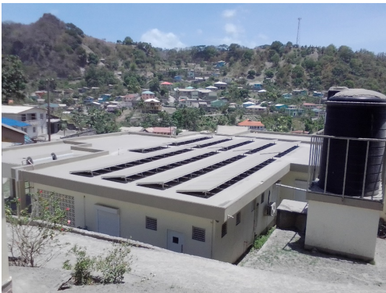
Chateaubelair Clinic rooftop covered in ash. Picture taken 28 th April 2021 by Mr. David Latchman
