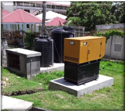
Image 2 - Outdoor genset with large capacity built-in fuel storage bolted onto RC plinth
