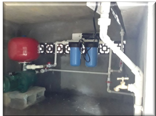
Image 3 - Pump with pressure tanks installed in existing pump room.
