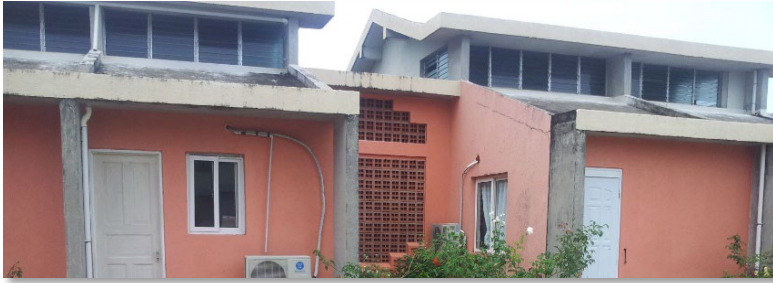
Image 3 - Glass louvre windows are high risk to falling, breaking and causing injury
