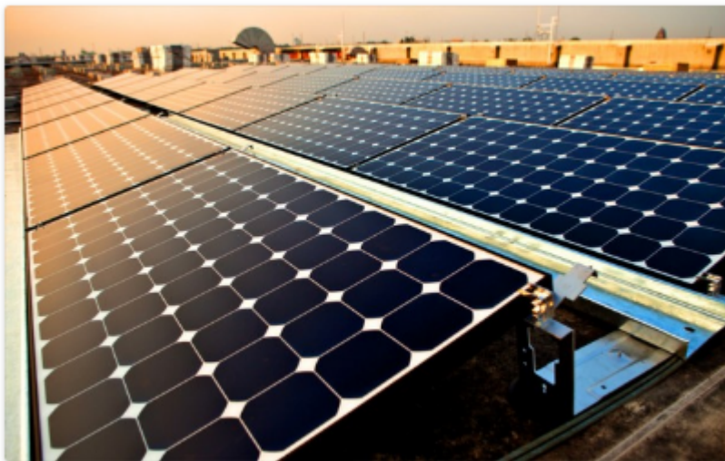
Figure 5 : Roof-Mounted Photovoltaic Panel Array (Aggarwal, 2018)
