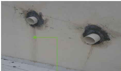
Water stain under drainpipe along face of wall
