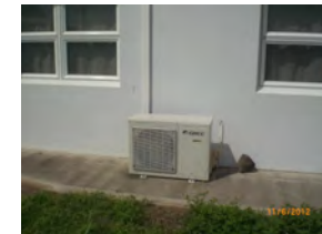
Split unit compressor on walkway next to emergency exit stairs
