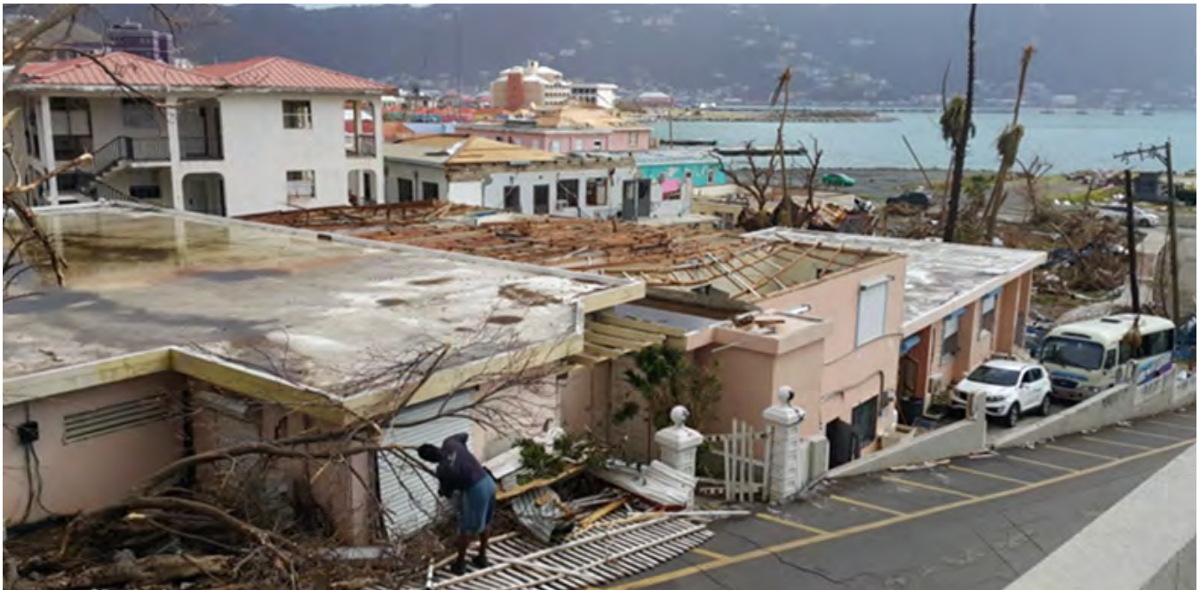
Photograph 1: Roof Damage from Hurricane Irma
