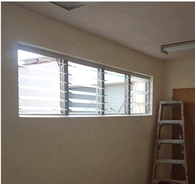
Photograph 4 Damaged Louvered Window
