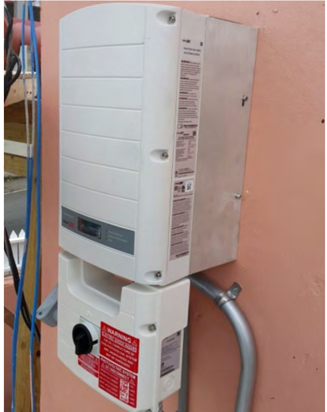
Photograph 15 PV System Inverter
