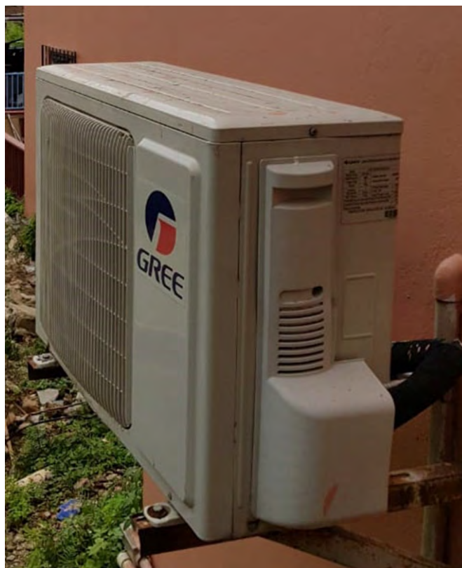
Photograph 18 Typical Inverter Type Split Unit Air Conditioning Installed
