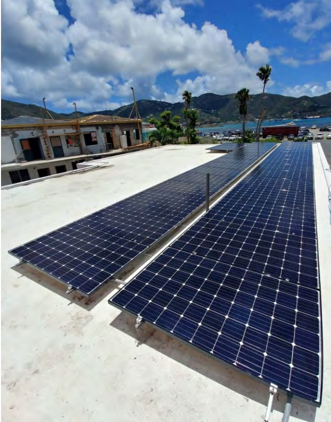
Photograph 14 Photovoltaic System Installed
