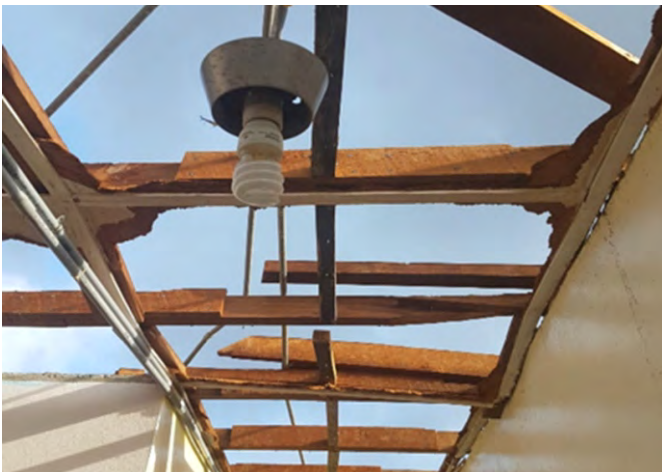
Photograph 16 Former Typical Light Fixture with Fluorescent Bulb
