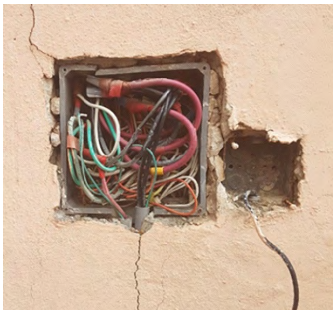
Photograph 7 Missing Electrical Covers
