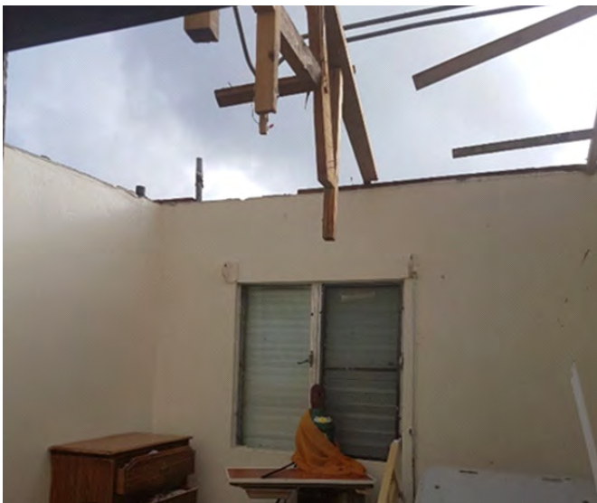
Photograph 2: Damaged Roof Members
