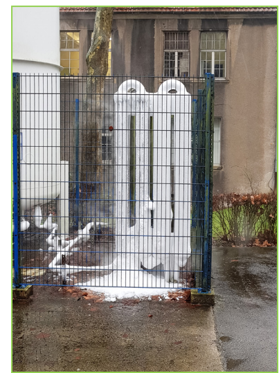
Image 8: Gasifier with ice on the outside.
