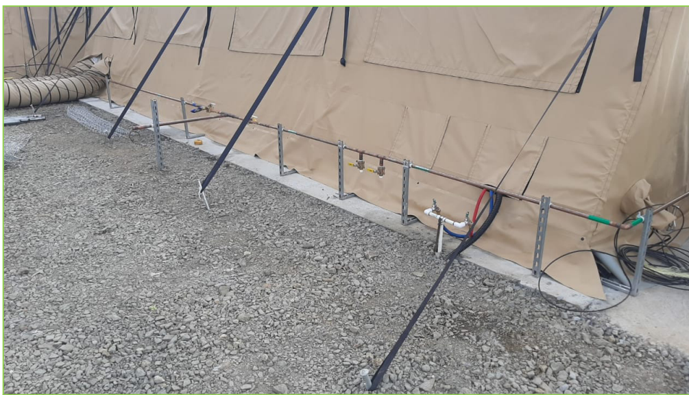
Image 3: Copper oxygen piping on the outside of a tent. The pipes are marked in green and fixed with metal supports. They are elevated from the ground and set under the tent's guy wires to avoid impacts (EMT SARI CSS Panama).
