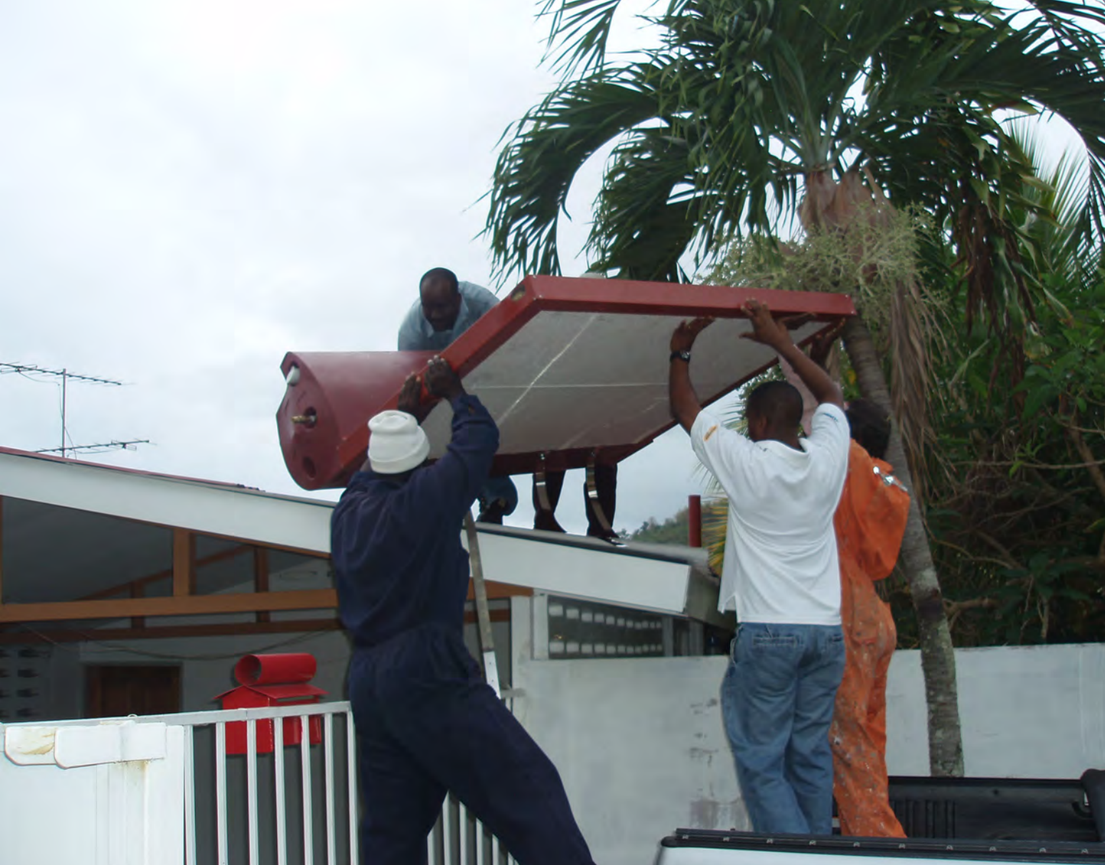
Residents install a solar water heating system on a house. Source: UNDP Trinidad and Tobago
