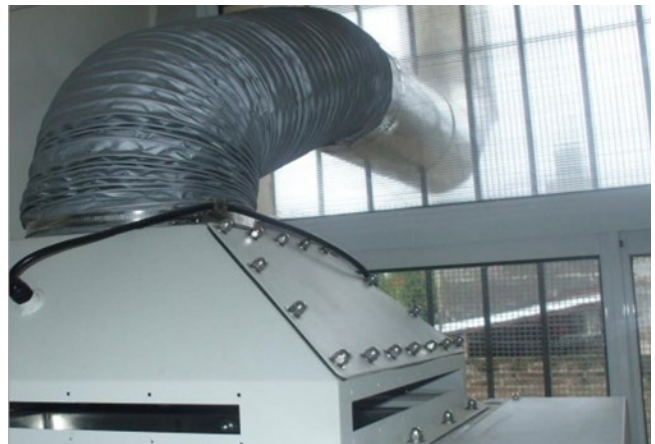
Duct connected in thimble on Class II type A biological safety cabinet that generates negative pressure
