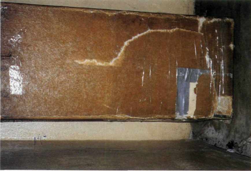
9. Fibreglass product box in poor condition.
