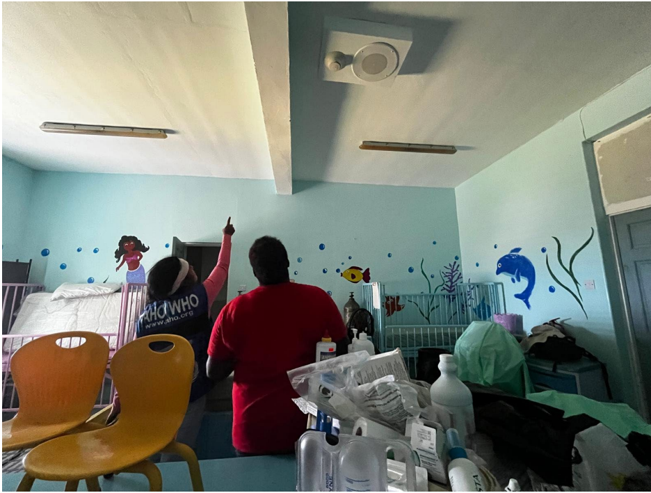
Examination of leaks at the pediatric room in Princess Royal Hospital, Carriacou
